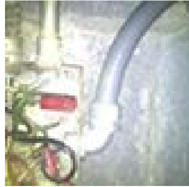
10-5h Shabby contractor work
