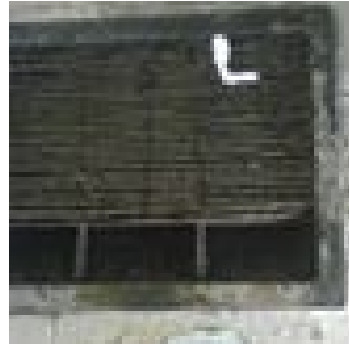
10-3h Air vents affect air quality
