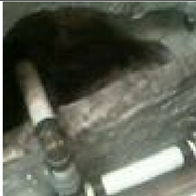
10-2e Hole in wall to water line
