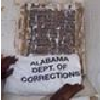
10-3g Vent in need of cleaning
