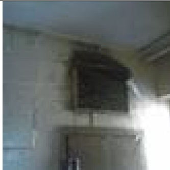
10-2a Air vents covered in mold
