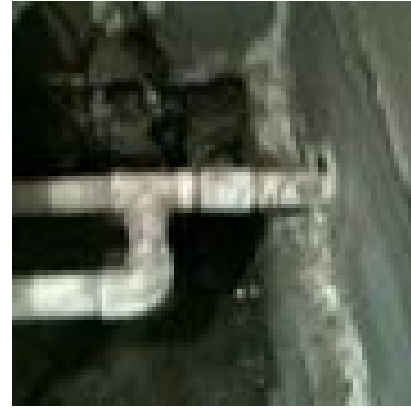
10-3b Corrosion in kitchen
