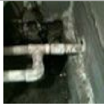
10-4b Corrosion in kitchen
