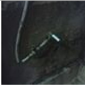
10-4a Contaminated water line
