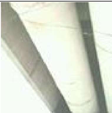
10-6c Kitchen roof falling apart
