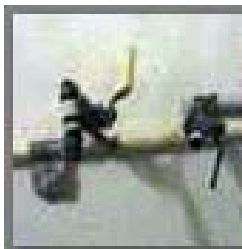
4h Broken shower head
