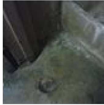
10-4f Mop closet mold enters living area
