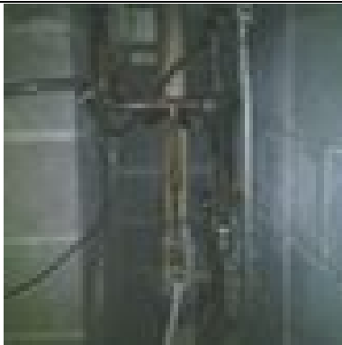
10-4g Nightmare inside pipe chase. Smell emits to cells
