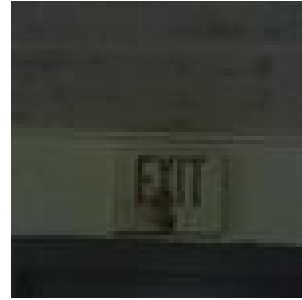
10-2d Fire exit broken and inoperable
