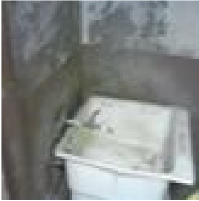
10-3a Another mop closet in disrepair
